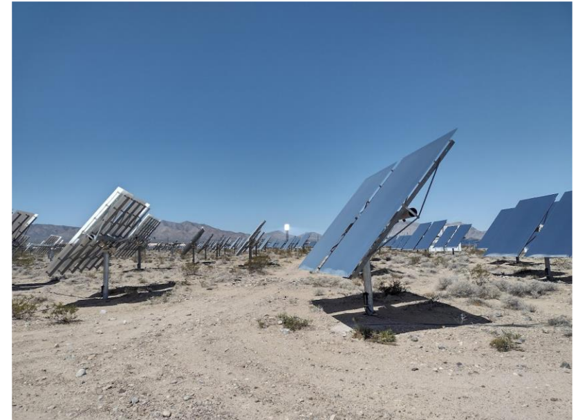
Heliostats in Ivanpah Solar Field, Unit 1
